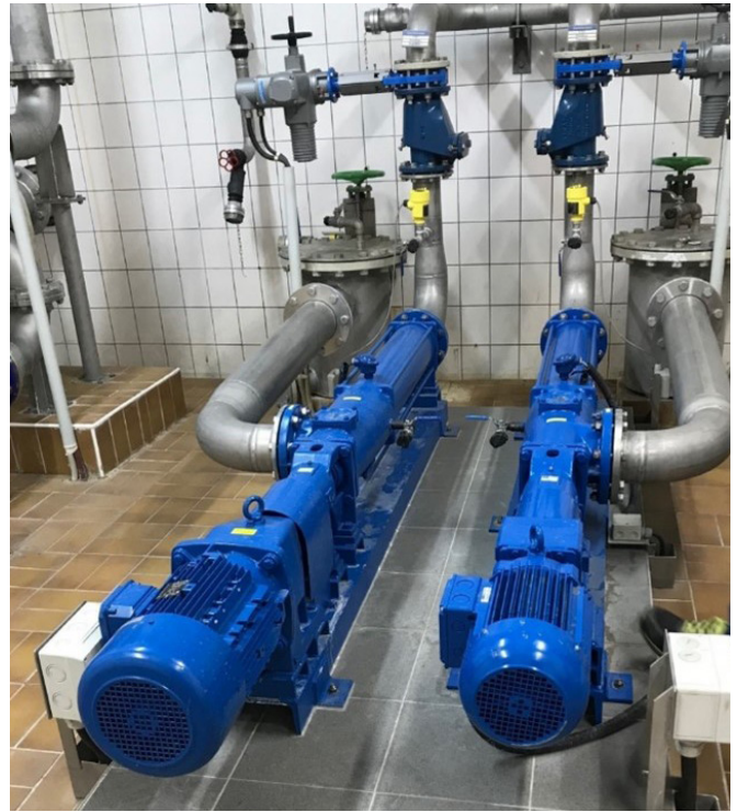
Two identical Allweiler PC Pumps of the type AE2E 750. They redundantly pump primary/raw sludge (6 - 10 m 3 /h at 61 to 97 rpm).
