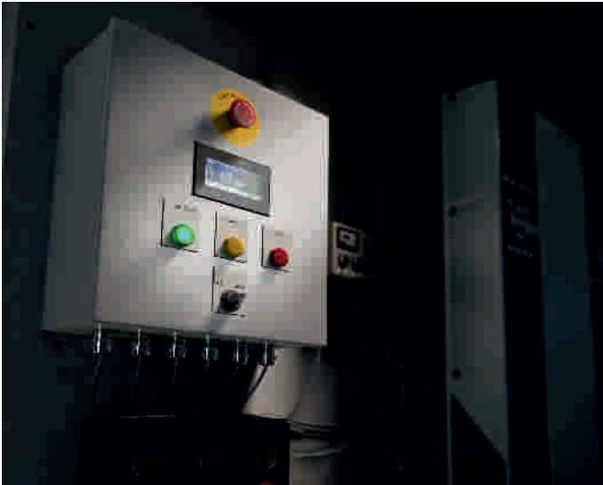
CM-1000 module installed in engine room.
