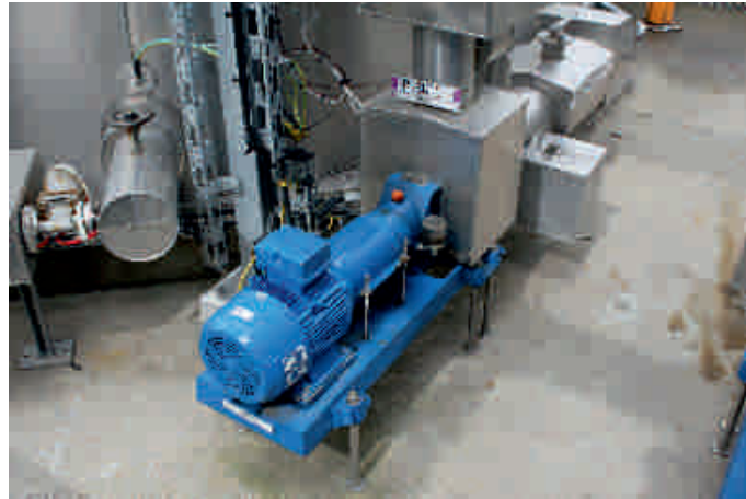
Series CNH-B 40-160/11 G-W20, capacity 20 m 3 /h, Liquid Farmin DM20, process: tank storage discharging.
