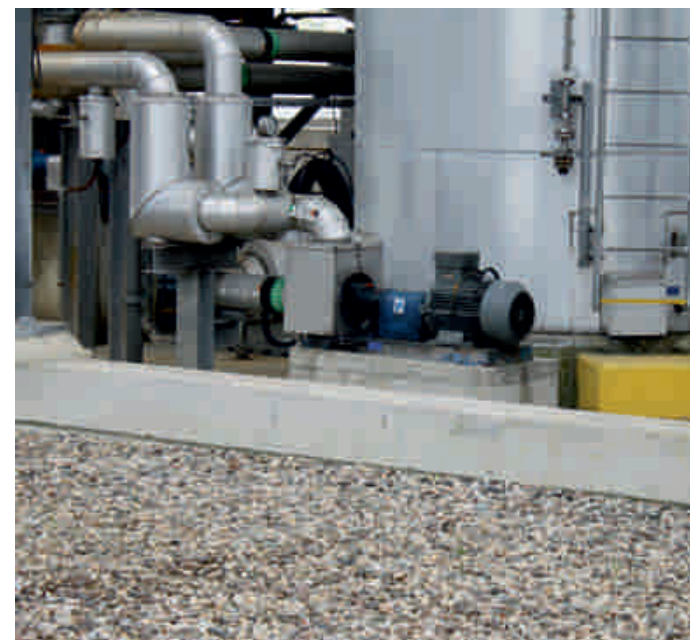
Series CNH-B 50-200G-W20, capacity 60 m 3 /h, liquid glycol/water, process: cooling system.
